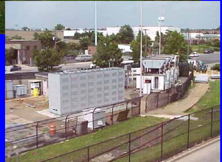
Three 600-HP compressors + 1 MW NaS battery
