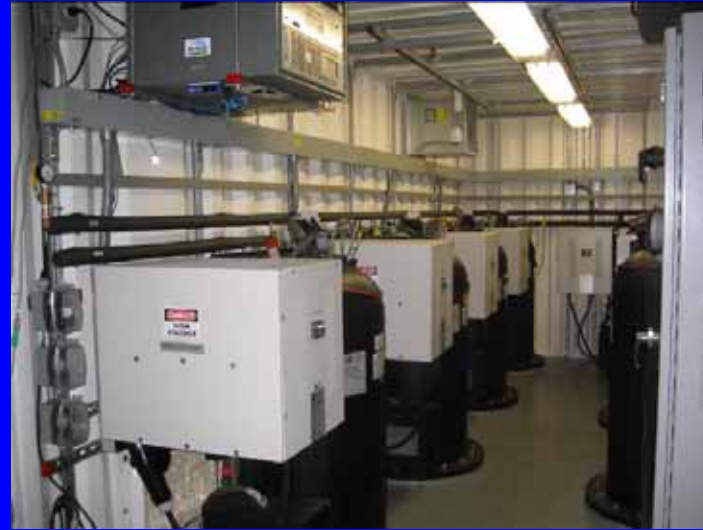
Containerized 7 Flywheel System
