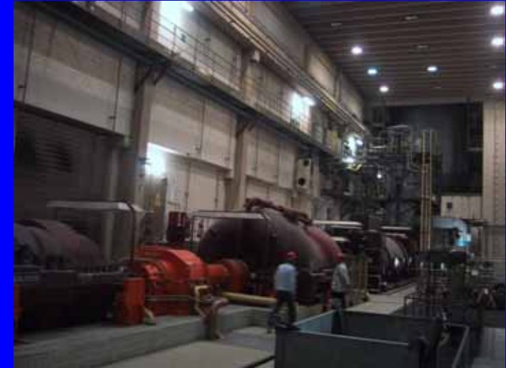
Huntorf, Germany, 290 MW
