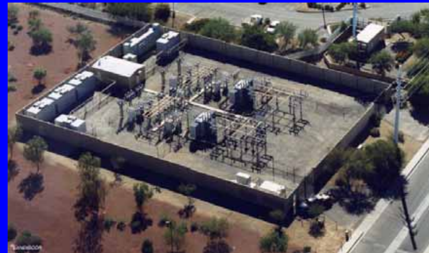
10 MW - 30 sec System at Microchip Plant
