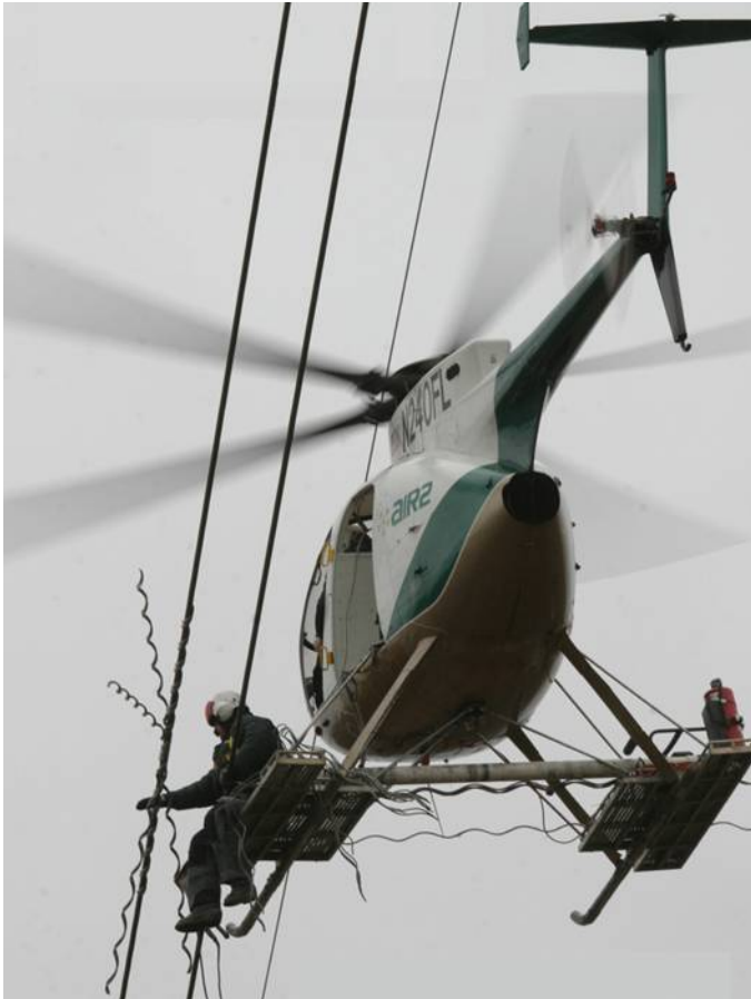
Helicopter Inspections Conducted in Spring & Fall – 1,620 miles of transmission lines inspected in 2004
